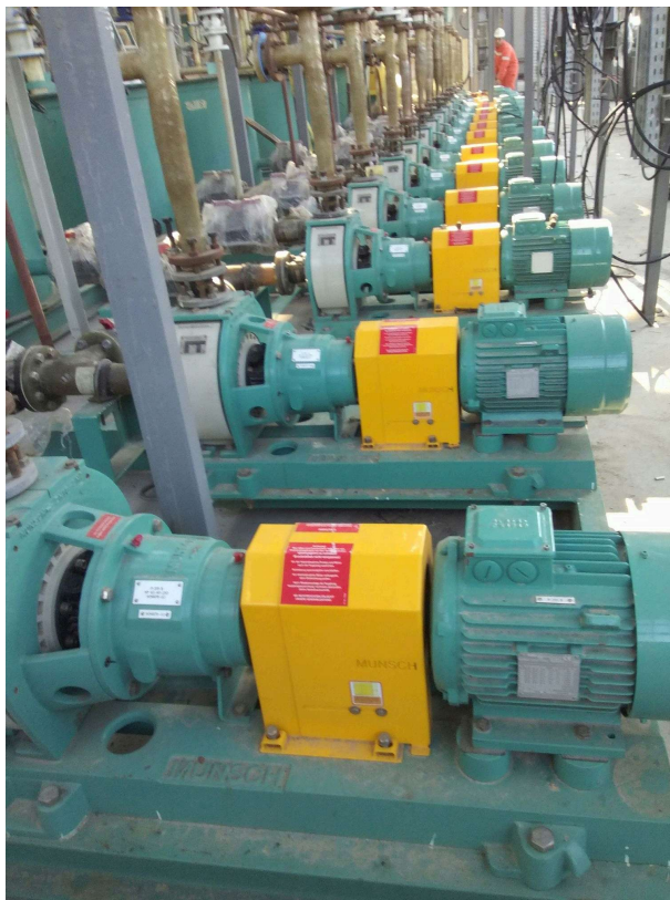
Pump skid forming part of INP's mechanical installation scope for gypsum / plasterboard works. INP Egypt LLC
